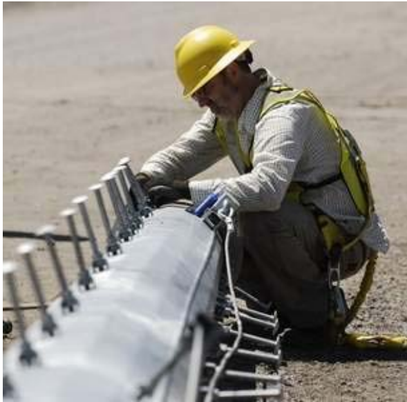
NO ROOM FOR ERROR: John Wakeman, owner of SUR Energy, double checks the wiring strung through the section before the crane lifts it Tuesday at Vantage Point in Port Huron. The top section slides onto the lower section.
